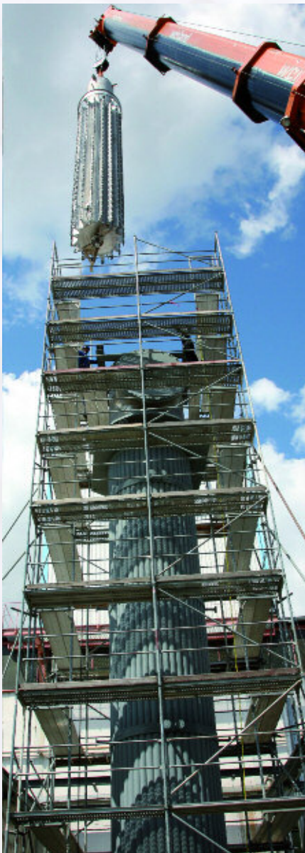
Assembly of CP dryer
